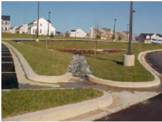
Curb Inlet #1: flow enters through curb channel.
