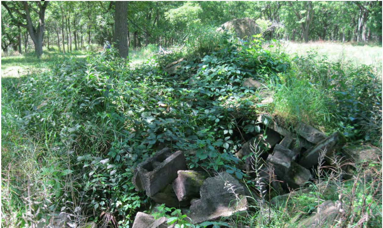
Photograph 2. Infilled poured concrete and "rock-faced block" foundation near STP 20.12, (shown in Photograph 10), facing west ( Panamerican 2015 ).
